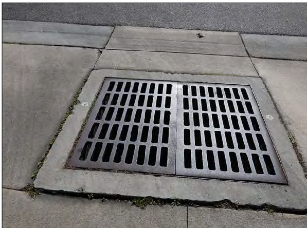
Stormwater Drainage Grate Inlet
