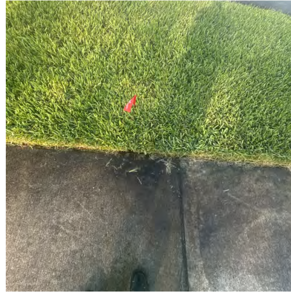
Zone #19 (Blocked Head) - 03-24-26 8:18 am CDT
