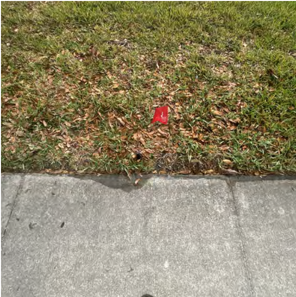
Zone #38 (Clogged Nozzle) - 03-24-26 9:46 am CDT
