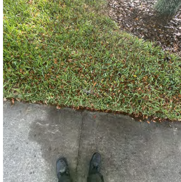
Zone #38 (Clogged Nozzle) - 03-24-26 9:46 am CDT
