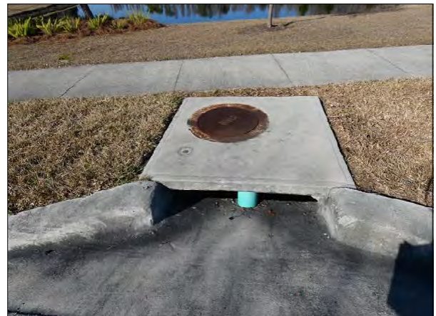
Stormwater Drainage Curb Inlet
