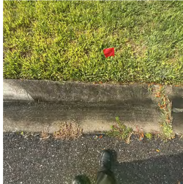
Zone #32 (Broken Lateral) - 03-24-26 9:22 am CDT
