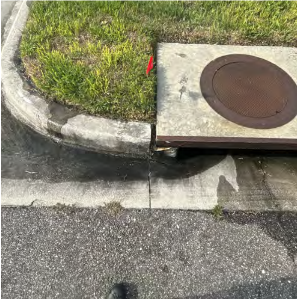
Zone #32 (Broken Lateral) - 03-24-26 9:22 am CDT
